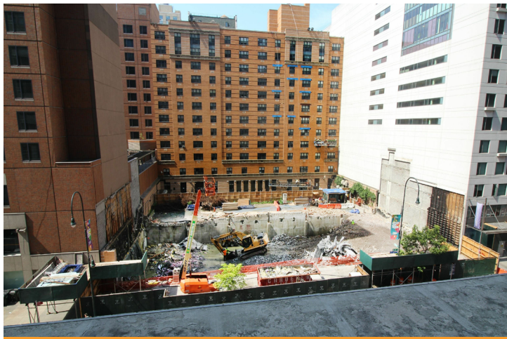
Recent progress at the Union Square Tech Training Center site, 120 East 14th Street
