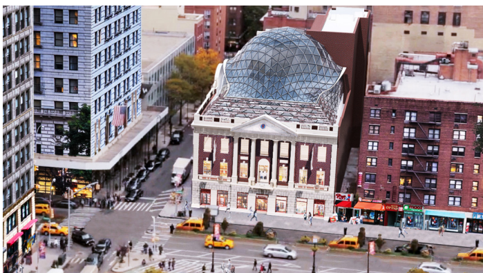
Restoration of 44 Union Square, designed by BSKS Architects, included the addition of a multi-story glass dome atop the 90-year-old structure.
